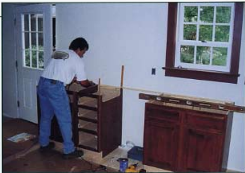
Rich also installed the cabinets for the small kitchenette on the wall opposite the fireplace. ▲
